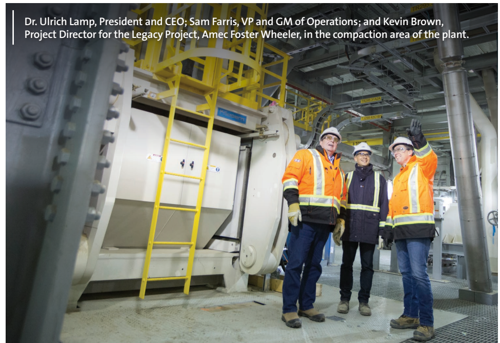
This 15-megawatt gas turbine electrical generator on site recently became operational.
